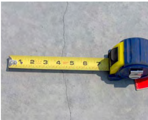
Typical Crack Width Opening With Wire
